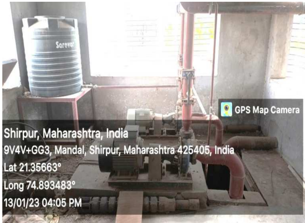
Water Conservation facilities at Institute (Bore-well at premises)
