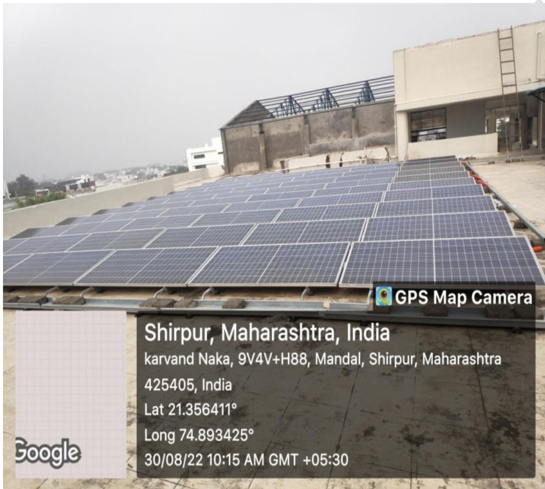
Solar Panel planted at roof of Institute.
